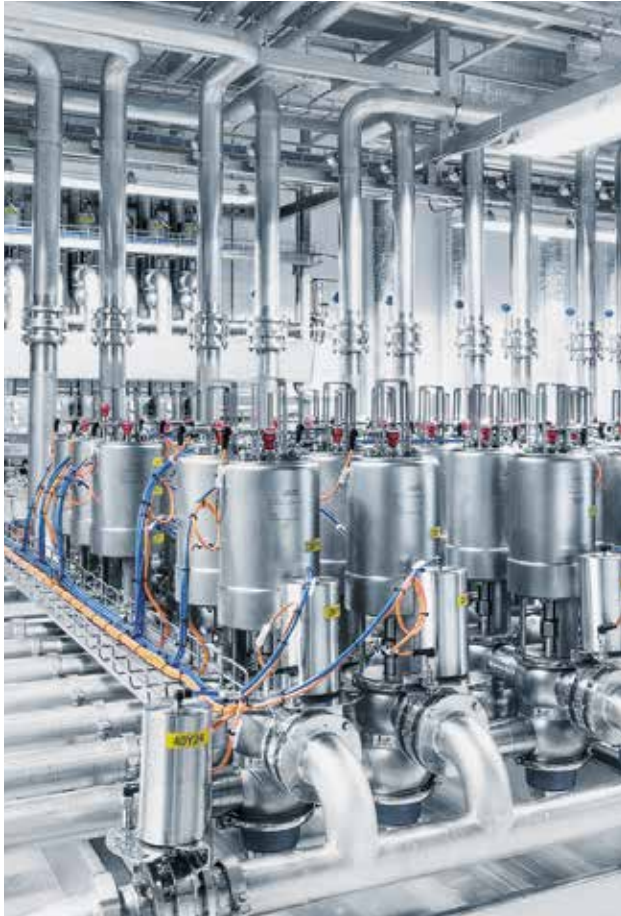
CIP valve manifolds
