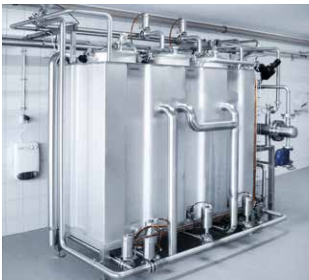
Cleaning station, cubic tank form
