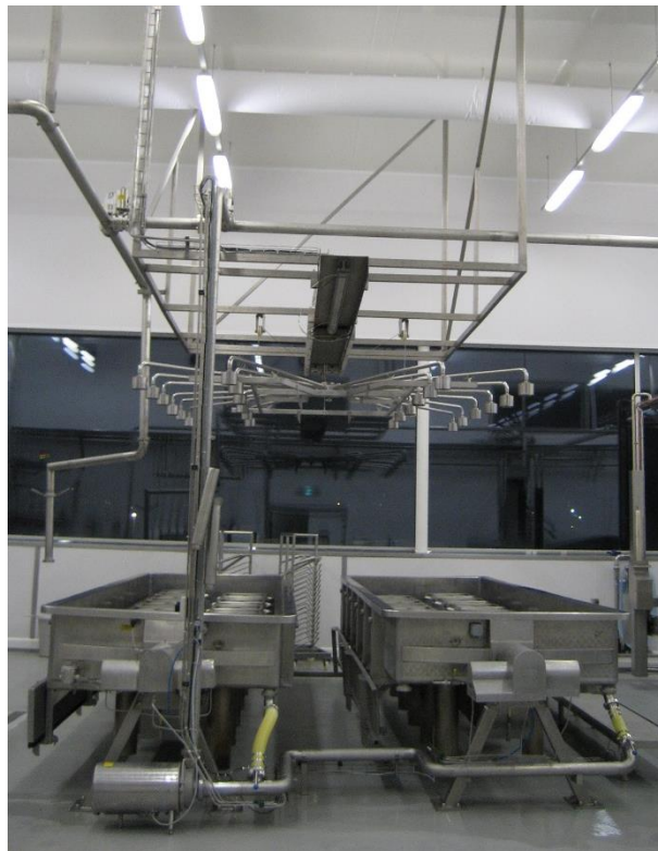
Integration of the existing presses into the new production
