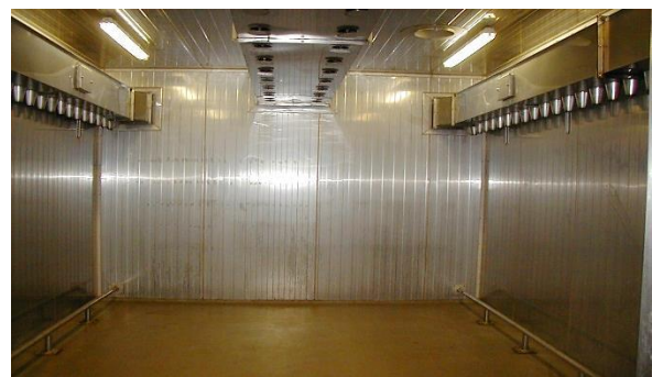
Cold smoke system
