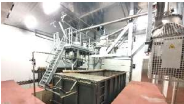
Automatic waste transport system
