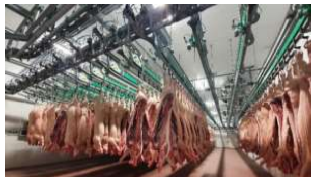
Automatic buffer cooling room
